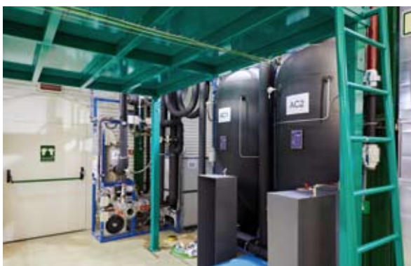
Fig. 2.5: Radon abatement system
