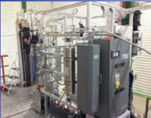
NEXT Gas System
