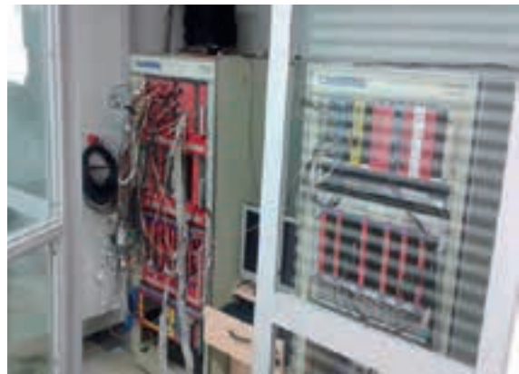
Fig. 5.1: ANAIS electronics inside a temperature-controlled space at LSC Hall B.
