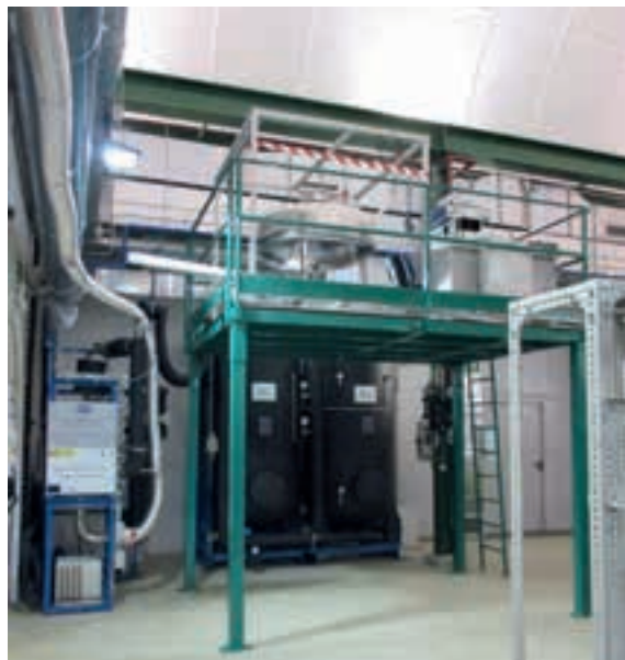
Fig. 2.6: New platform for radon detector
