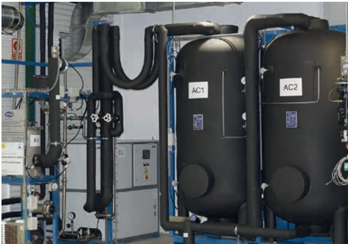
Fig. 2.3 Radon abatement system installed at LSC.
