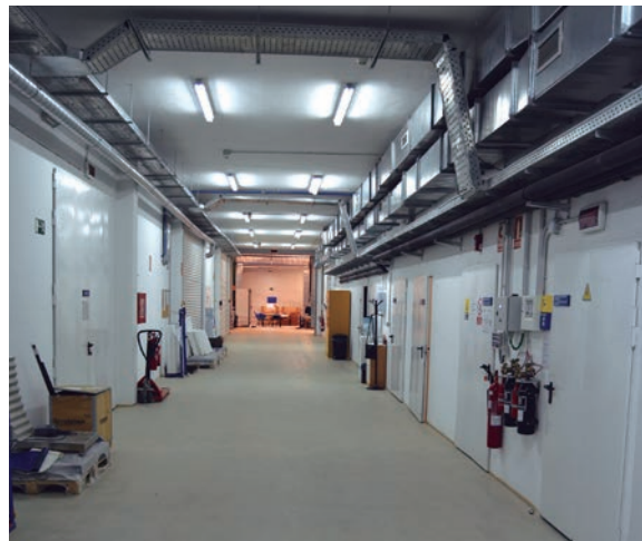
Fig. 4.7. The service aisle
